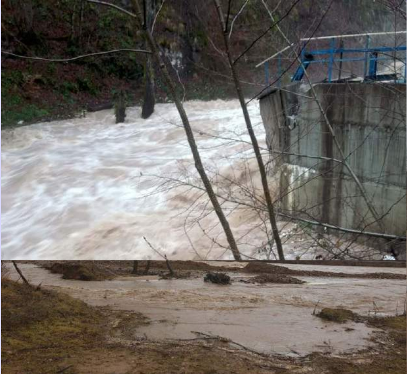
A strong flood shaved the dam of the Ştei water intake on February 4, 2020
